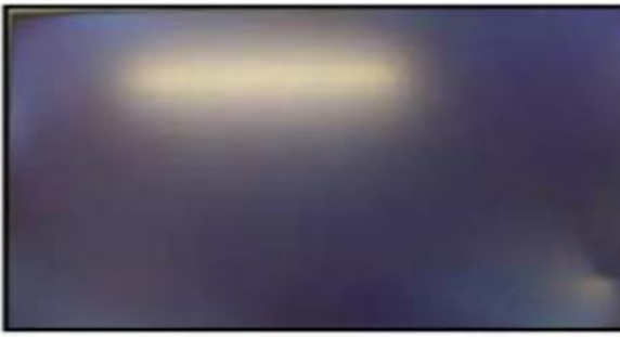
Fuse Open, Abnormal power section
